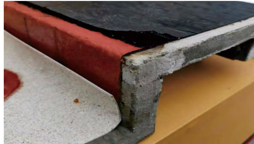
Waterproofing Membranes made of different materials are incompatible and cannot be compatibly sealed.
