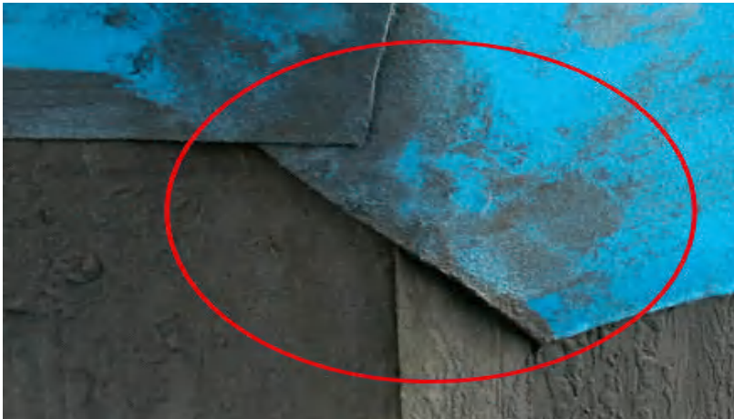
Common roof waterproofing materials and side - wall waterproofing materials are incompatible and cannot form a continuous and seamless whole.
