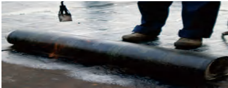
Construction cannot be carried out on a damp base surface, and it's difficult to bond and seal with the base surface on - site.
