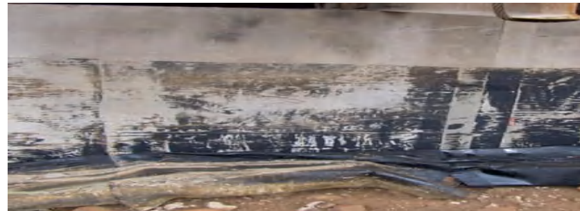
Self - adhesive Waterproofing Membranes can't maintain a long - term bond with the base surface.
