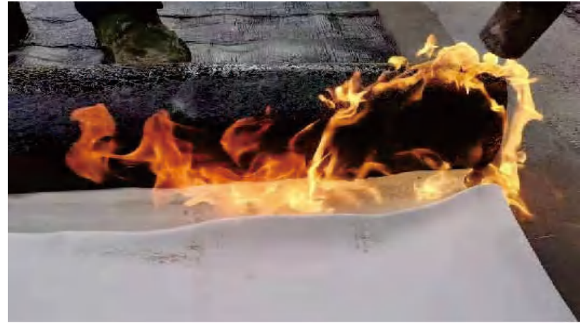
The hot - melt torch - heating of SBS waterproofing rolls may damage the underlying polymer rolls.
