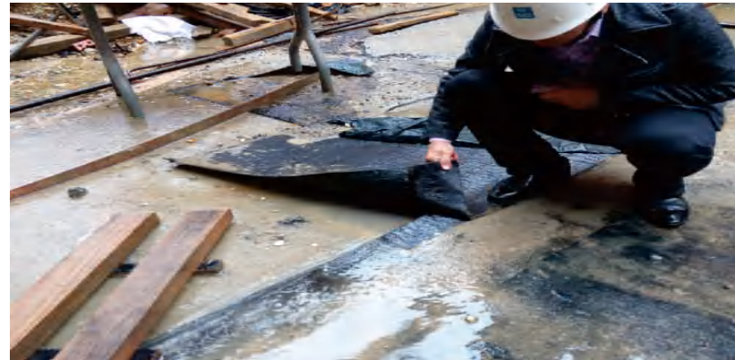
Traditional Waterproofing Membranes can't adhere to the on - site concrete substrate.
