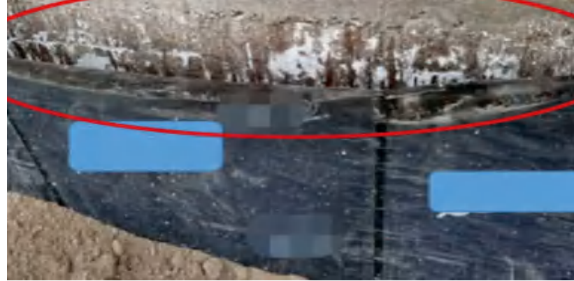
Temporary adhesion and false sealing pose even greater damages.
